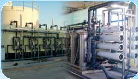
PUBLIC ELECTRICAL ENTERPRISE OF RHODES/GREECE
