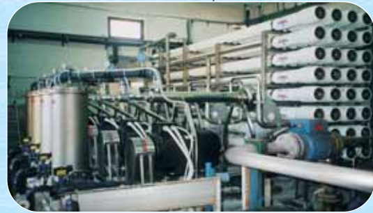
WATER SUPPLY AND SEWERAGE CO OF ERMOUPOLIS/GREECE
